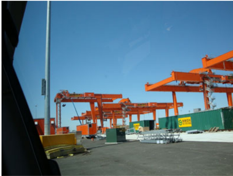
Figure 1 - New Intermodal Cranes Under Construction at the BNSF Intermodal Facility, Memphis, TN
