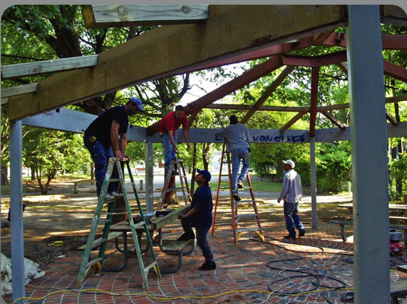
Construction of a gazebo in a park in the heart of the Pigeon Roost / Annesdale community.
