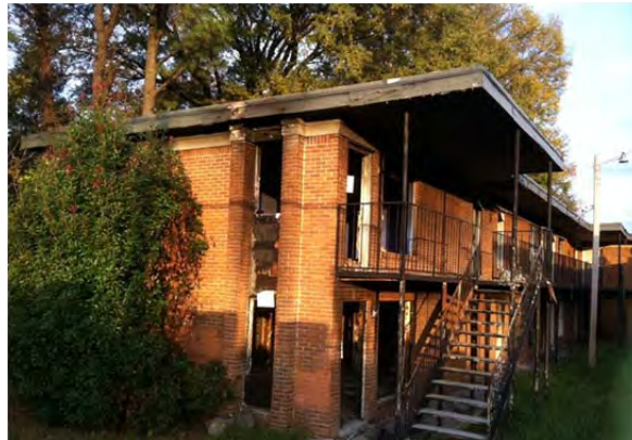
Image 3: This 10 to 12 unit “shoebox” apartment building, typical of many found throughout Memphis, often on formerly single family lots, has been abandoned because there is no current market for it in its neighborhood.
